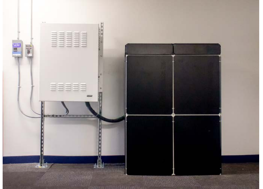
Power Assurance demonstration system at UEP headquarters
