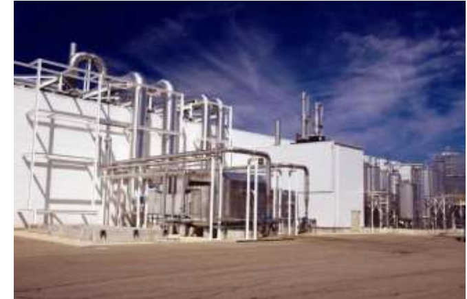
NMP Recovery & Purification
